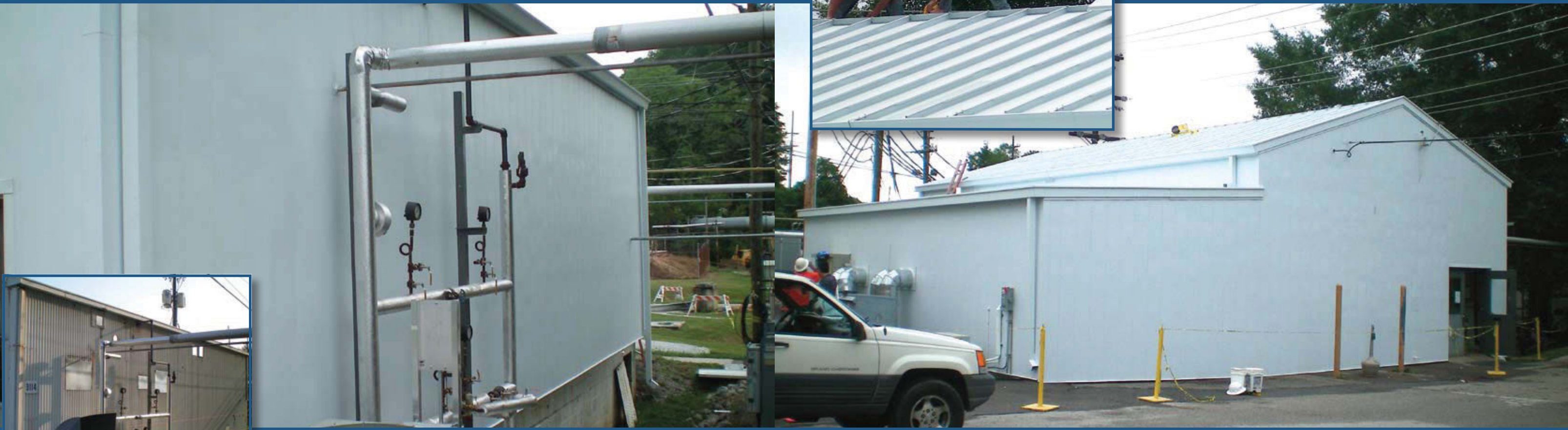
Inset: Before Paramount's involvement, the south side of this building at Oak Ridge National Laboratory was thermally inefficient with a number of penetrations. Main photo: After Paramount completed the retrofit, the thermal efficiency sharply increased.
